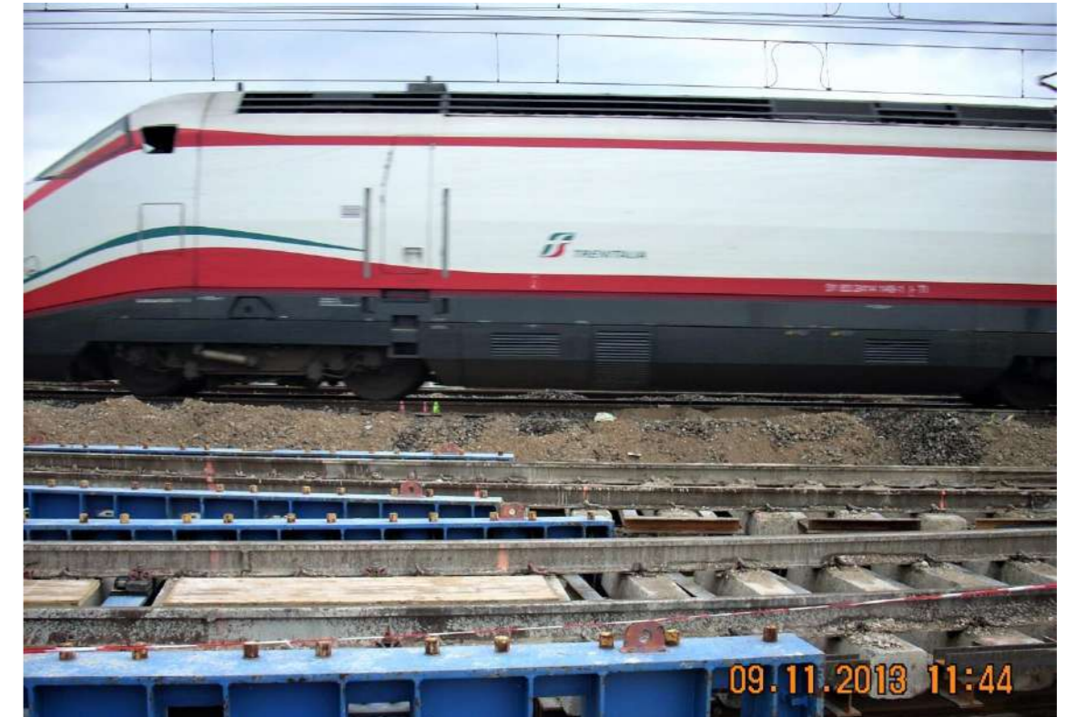
Figure 4 - Active traffic flow during Box Jacking works which shows the great difference in height between the tracks
