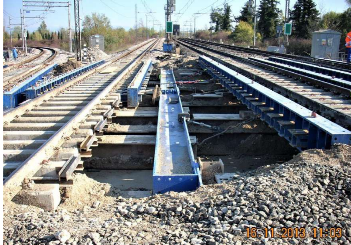
Figure 5 - Verona System installed on tracks that are placed at different levels
