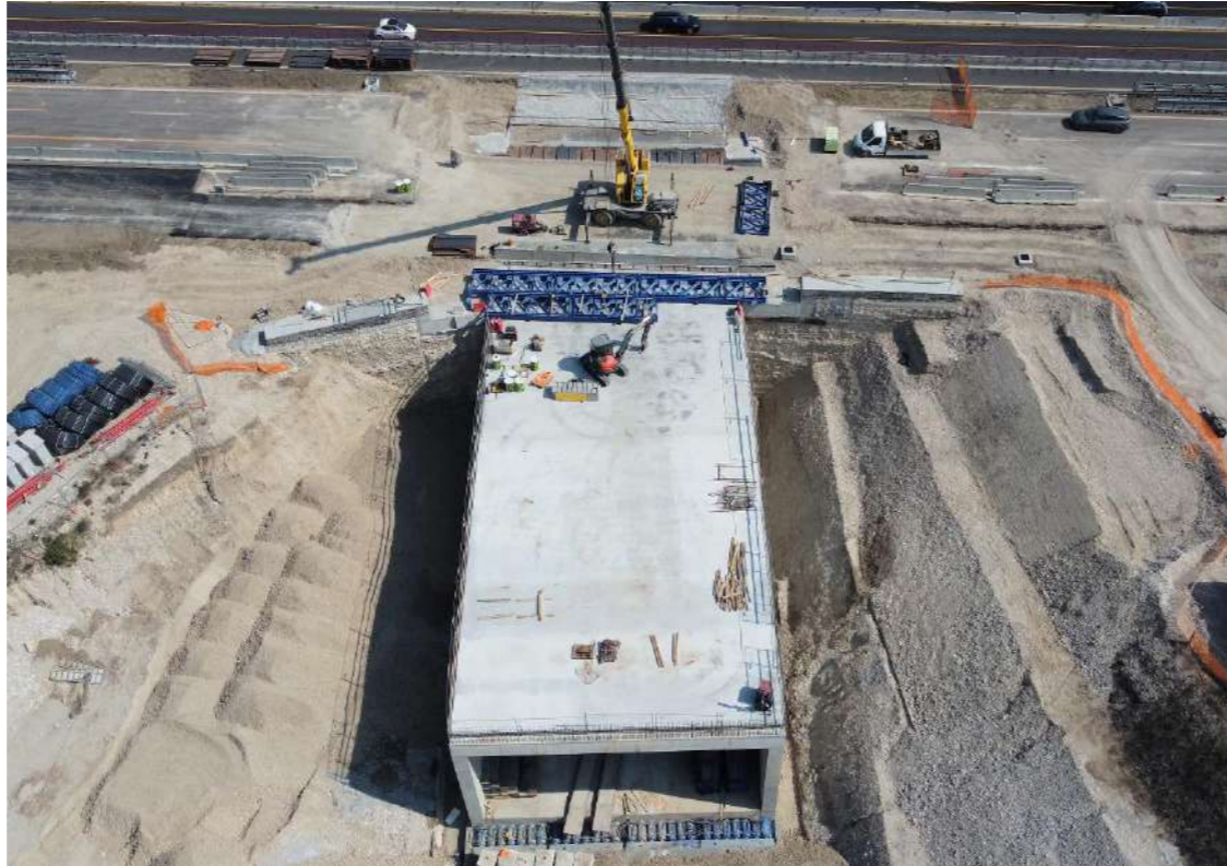
Figure 5- Restraining beam of the Anti-drag system installed on MS3E013
